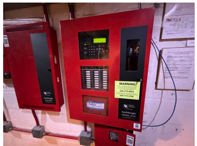
18 - FIRE ALARM PANEL
