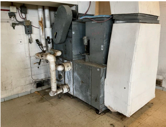
15 - TYPICAL AIR HANDLER
