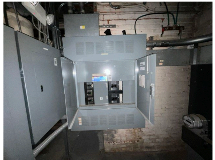
16 - MAIN DISTRIBUTION PANEL
