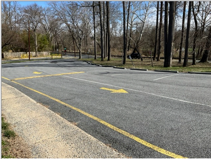
NO ADA PARKING OBSERVED
